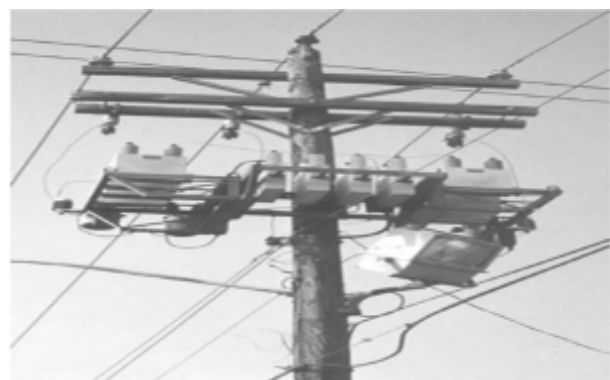
Fig. 2: Distribution capacitor bank
